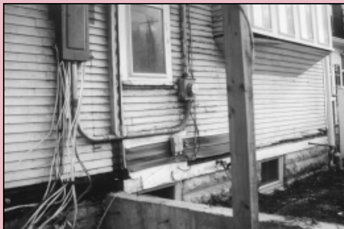
The original clapboard siding is revealed as the vinyl siding is being removed.
