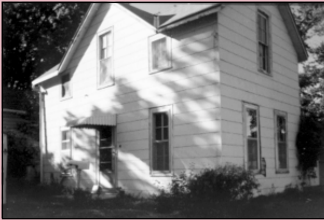
The Runyon House at 400 Osage in Manhattan is shown first with its asbestos siding and secondly after the removal of the asbestos and repair of the original clapboards.
