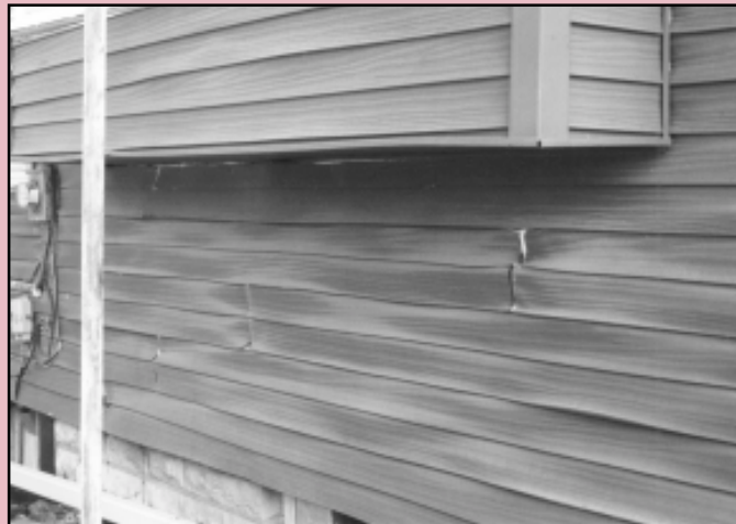
This photograph shows the warped vinyl siding on the rear of the Warren Wesley Finney House in Emporia.
